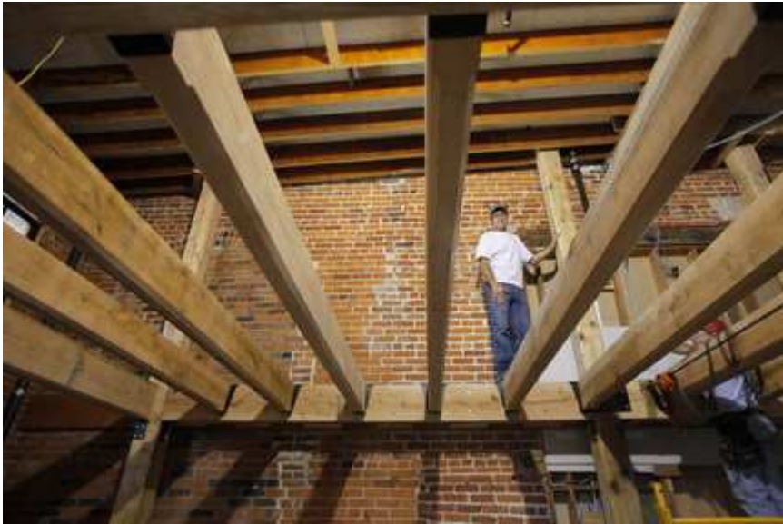
Mark Bugnaski / GazetteBalancing beam: Builder Rock Bartley stands on top of what will be the mezzanine in the new music room at Bell's Eccentric Cafe. Bartley also plays with the band Great Lakes Grass, which will perform at the 25th anniversary party.
